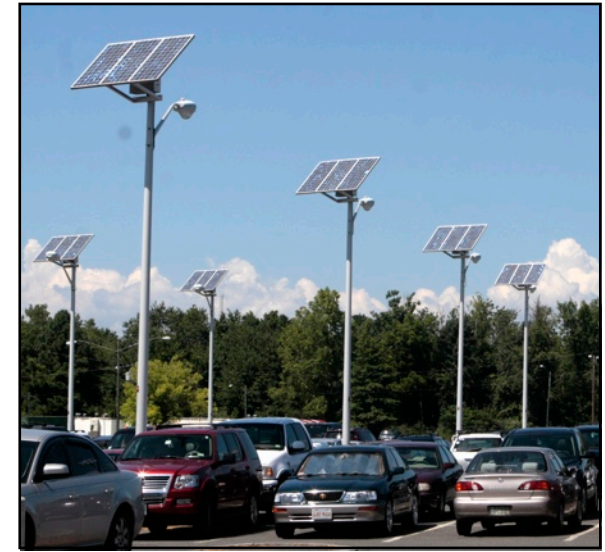
Solar panels power lights at the UMass Mullins Center parking lot
